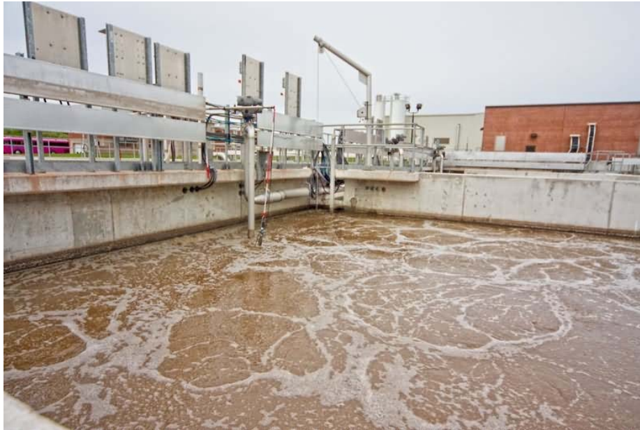
Figure #1 Aeration tank of Biological Nutrient Removal (BNR) System.
